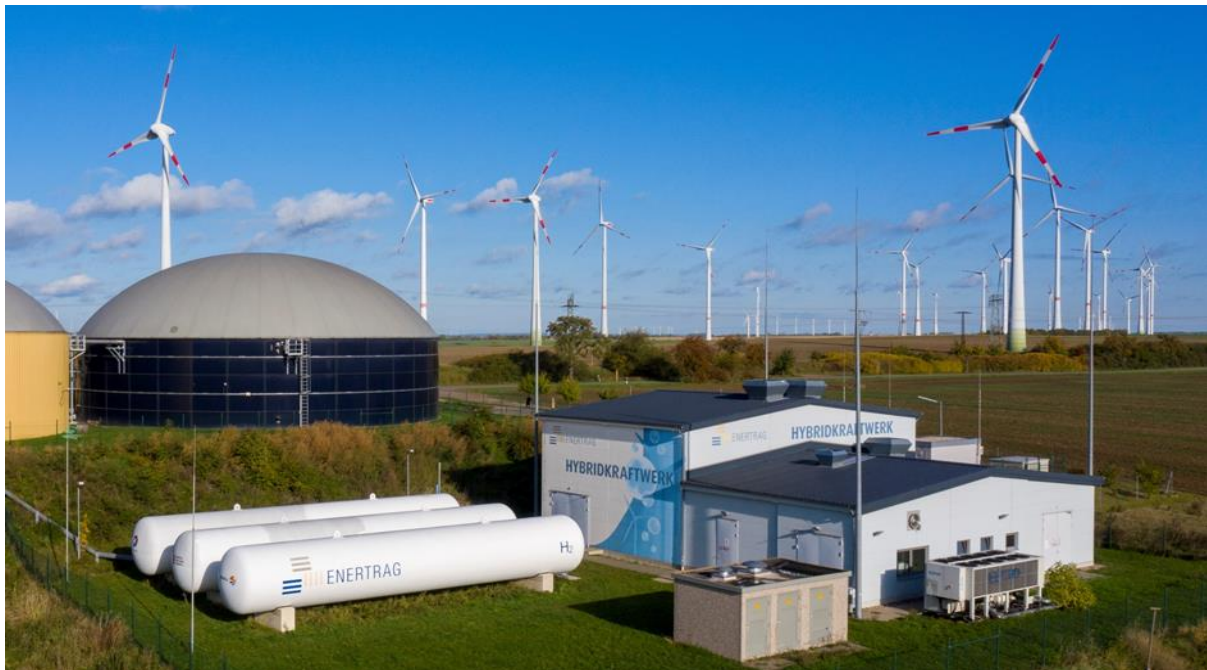
Figure 6-4: Closer View of Electrolyser Housing and Storage Tanks
