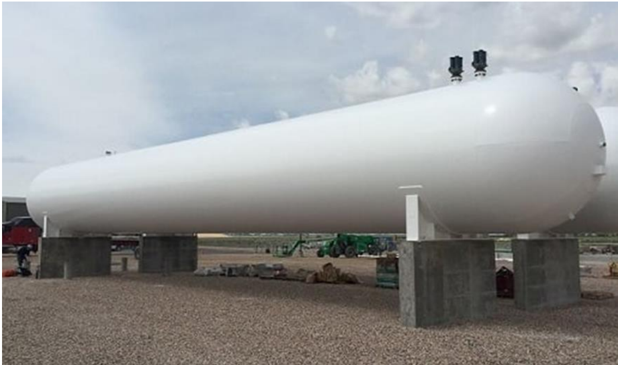
Figure 6-17: Bullet storage tank (ammonia/hydrogen storage)
