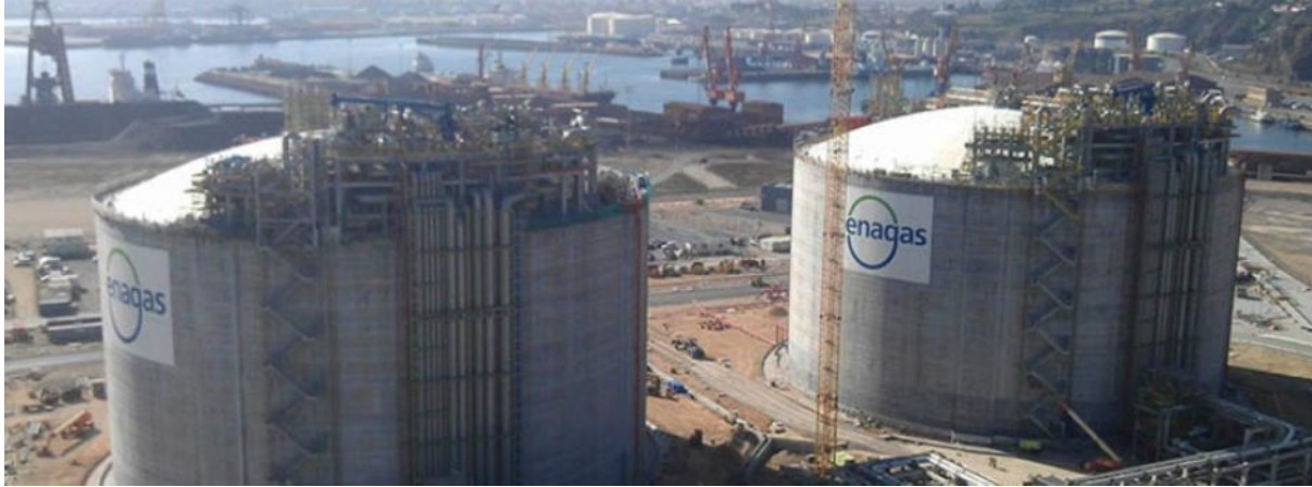
Figure 6-18: An example of a Liquid Ammonia Storage System (Source: Energas)
