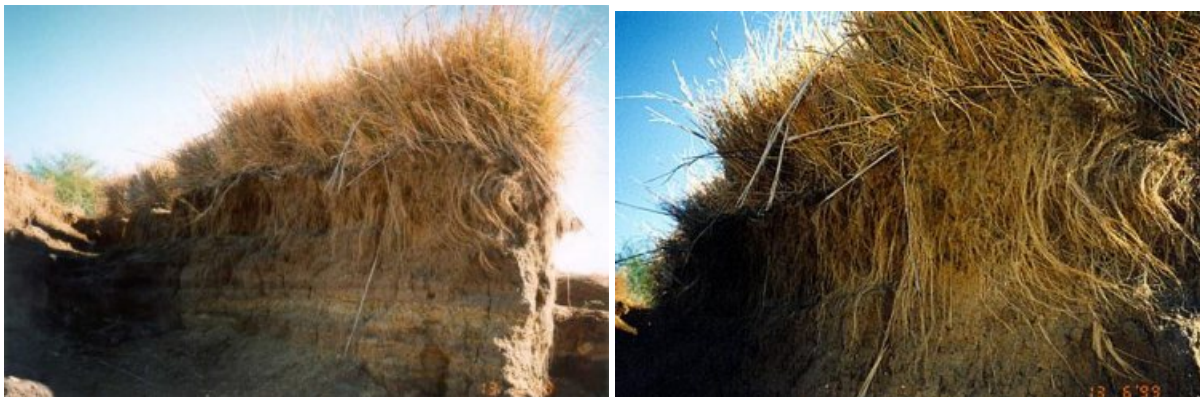
Strong root penetrating several layers of compacted dam wall
