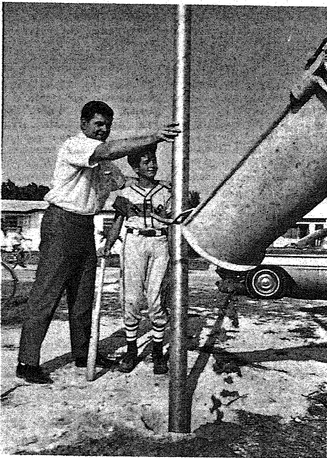
FIRST POST is set in place by contractor George Baumgartner for Holy Family parish's regulation pony league diamond while Anthony Devecchio, 12, watches the beginning of work that will be completed in four weeks. Funds for the new baseball lot were raised by the HD women's club.
