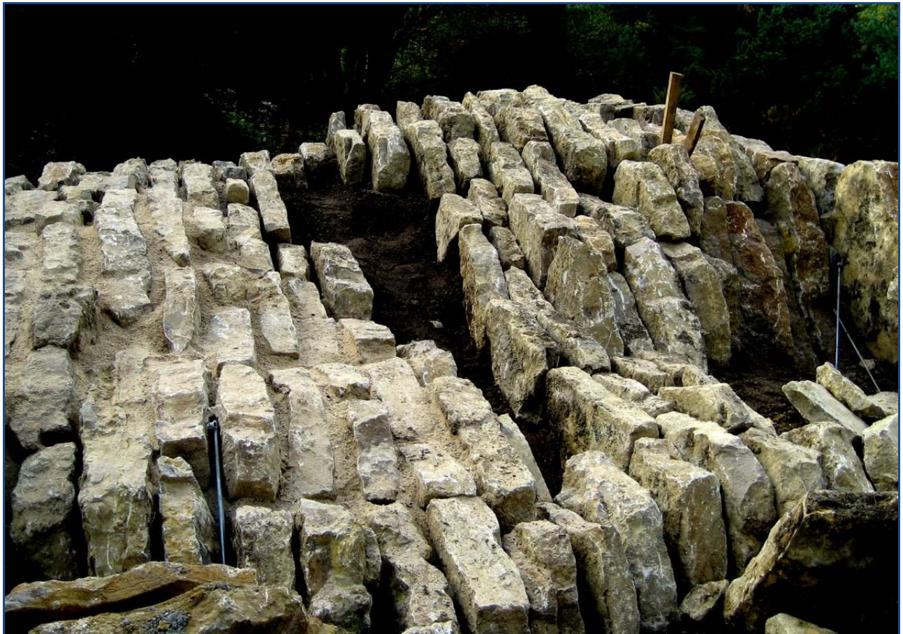
North-east slope under construction; body (underground) rather ‘mineralic’; crevice filling with a sand/pebble mixture.
