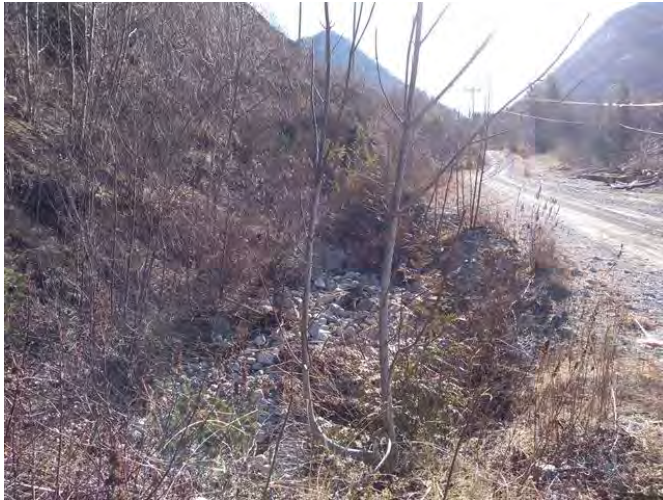
Photo 84: Looking east at Roadside swale along the Furry Creek FSR above Middle Creek Tributary 1. March 4, 2019.
