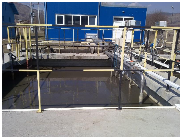
Figure 220 Wastewater treatment, Buzău (foto: Iulia Miu)
