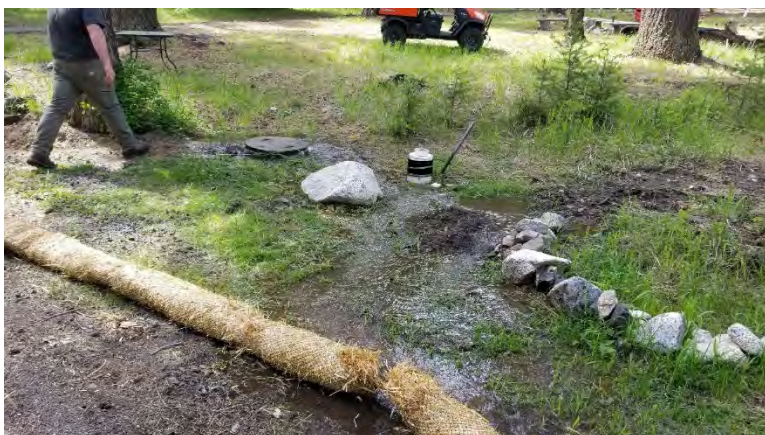
Photo 3: Septic holding tank pump vault cover: source of discharge
