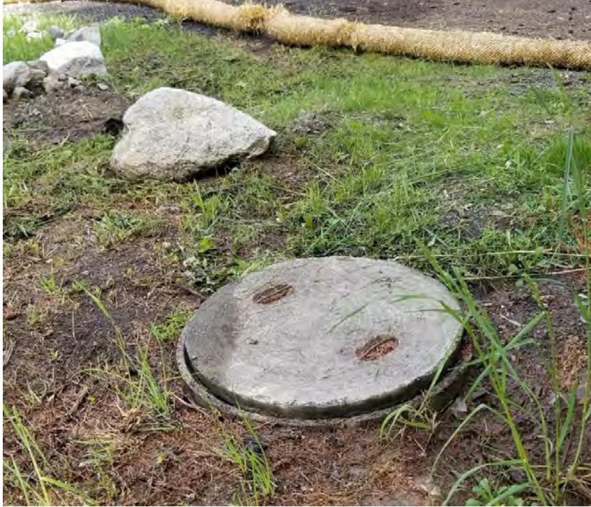
Photo 4: Discharge has stopped (June 3, 2020 at 11:47 AM)
