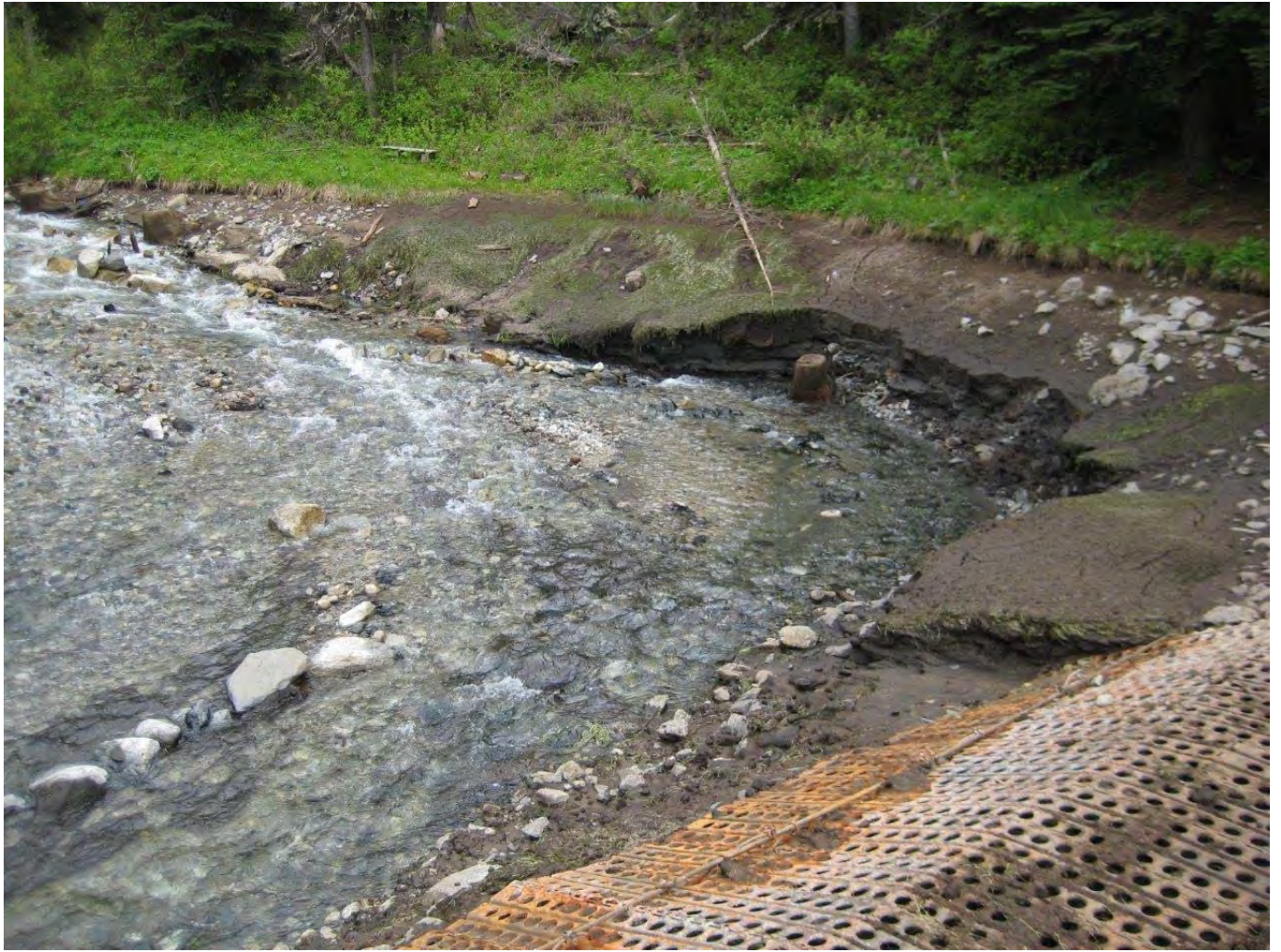
Photo 3 –Wallowa Falls Forebay – some sediment cutting along edges during draining on June 15, 2020
