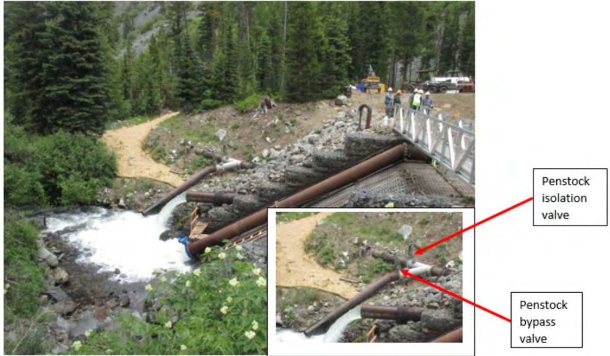
Figure 1: penstock wye with knife gate valves
