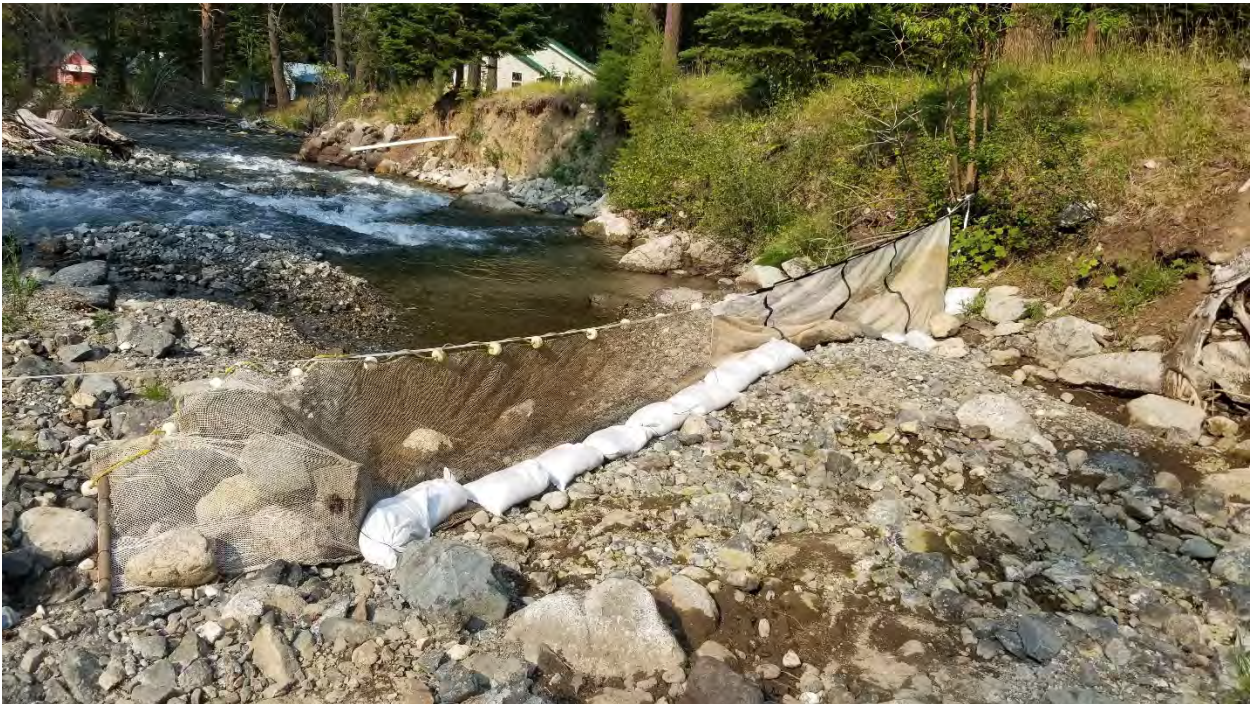
Figure 4. Photo of Wallowa Falls side-channel barrier at the downstream end.
