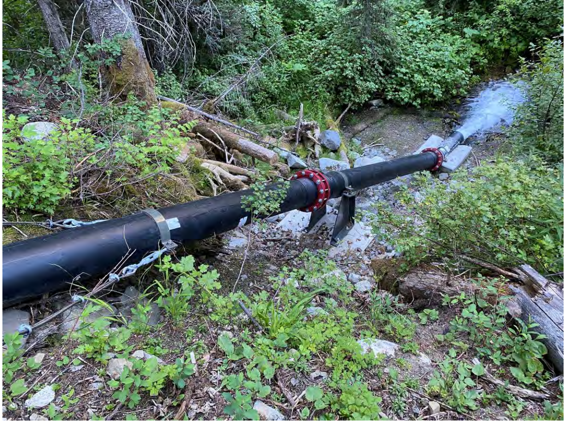
Figure 3. The discharge pipe from Royal Purple Creek installed 2019. (photo- July 27, 2020).
