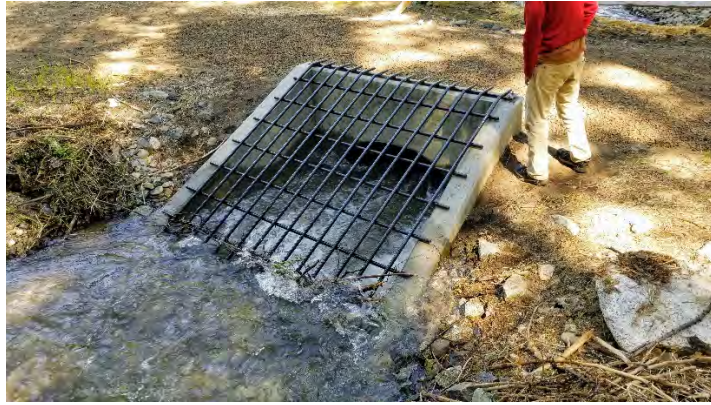
Photo 4: Trash rack upstream of road culvert on lower north tailrace channel (June 5, 2020)
