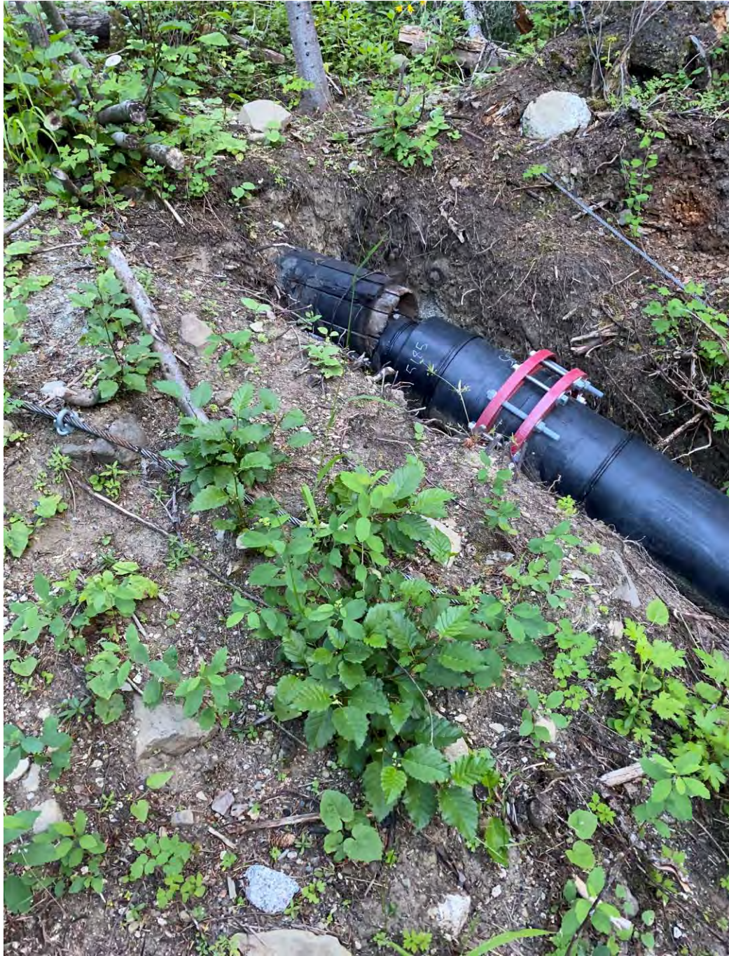
Figure 4. Junction of the existing and new discharge pipe from Royal Purple Creek. (photo- July 27, 2020).
