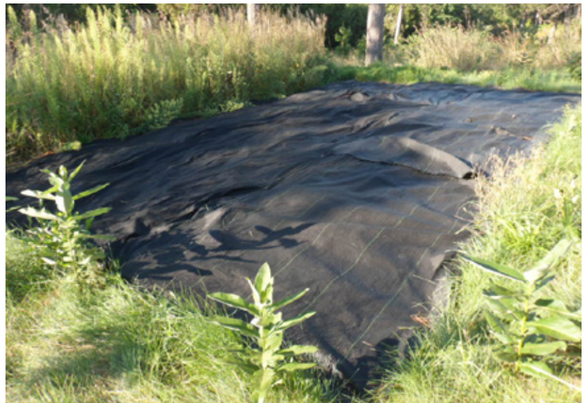
Tarping done by the City of Toronto using a black landscape fabric.
