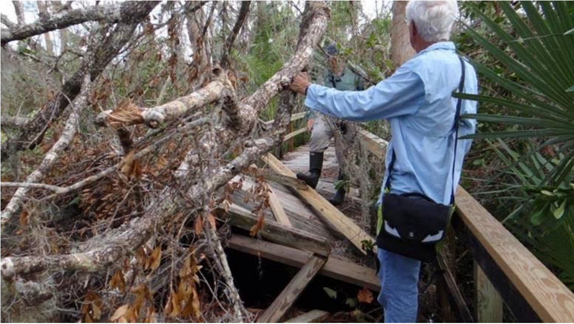
Damage from the root ball of a tree that fell away from the boardwalk.
