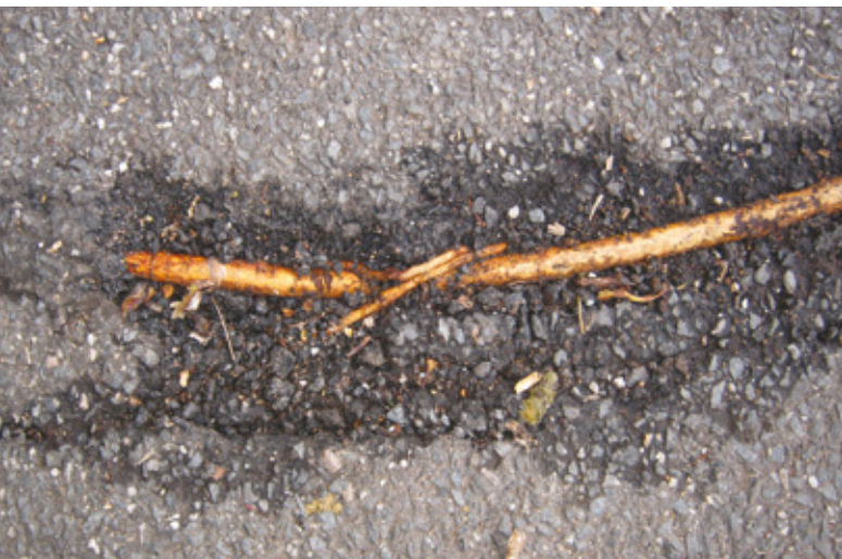
Plant roots can be very destructive, as shown by this image of tree roots causing severe cracks in bitumen paving. A root barrier on a green roof can protect the underlying layers
