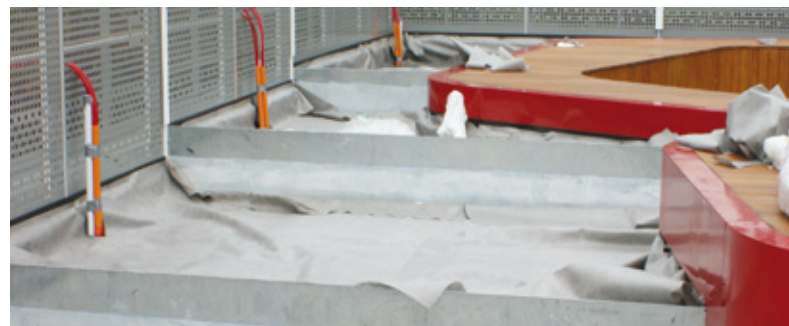
A layer of filter sheet will prevent substrate dropping into the drainage layer. Enough filter sheet is set down over the roof so that at the vertical edges of the planting beds the sheet will be the same height as the substrate
