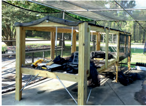
The old cutting benches of the BRCS were made from scrap lumber and after many years use were no longer servicable, so Art Hoover and Charlie Johnson are building a new one out of treated lumber. Almost finished, it just needs it's shade cloth cover. It will have a leaf valve to turn the water to the mist heads on and off. When the leaf dries off, it opens the valve and when it gets wet, it closes the valve.
