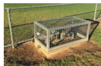
Water meter cage example
