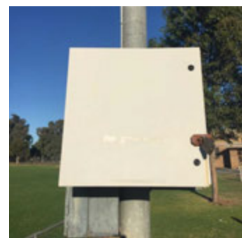
Irrigation cabinet example
