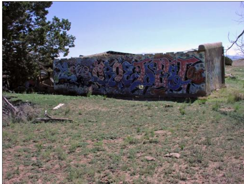
Figure 69. Early 20th century Forest Service administrative building near a dispersed camping area, painted with graffiti, Española Ranger District
