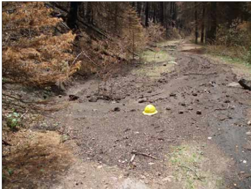
Figure 55. The Las Conchas Fire burned intensely uphill of this road, removing all vegetation and litter. After a storm, the runoff collected debris and impacted this road.
