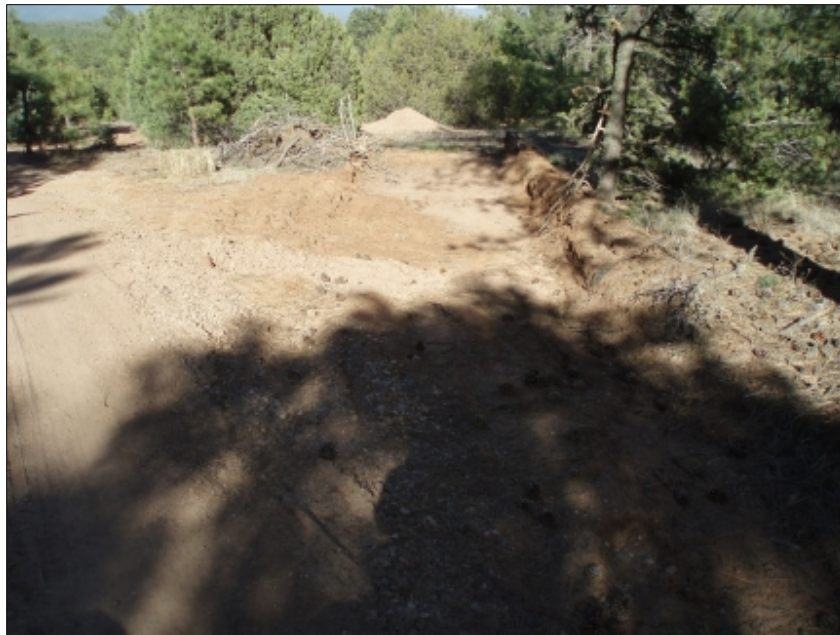
Figure 57. Example of a ditch that carries water off the road, so it prevents sediment from being carried to streams
