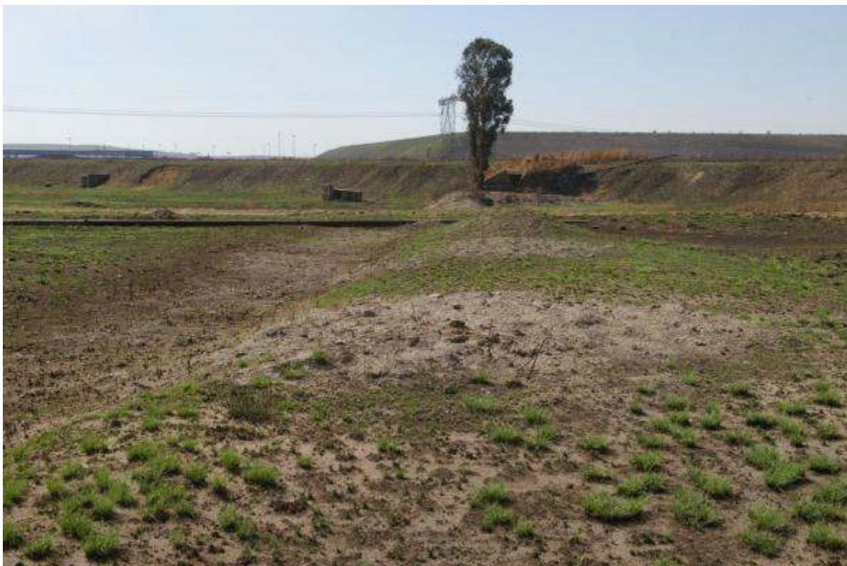
Figure 20. Broken farm dam wall and road crossing in the southern wetland unit. (Alternative 2)
