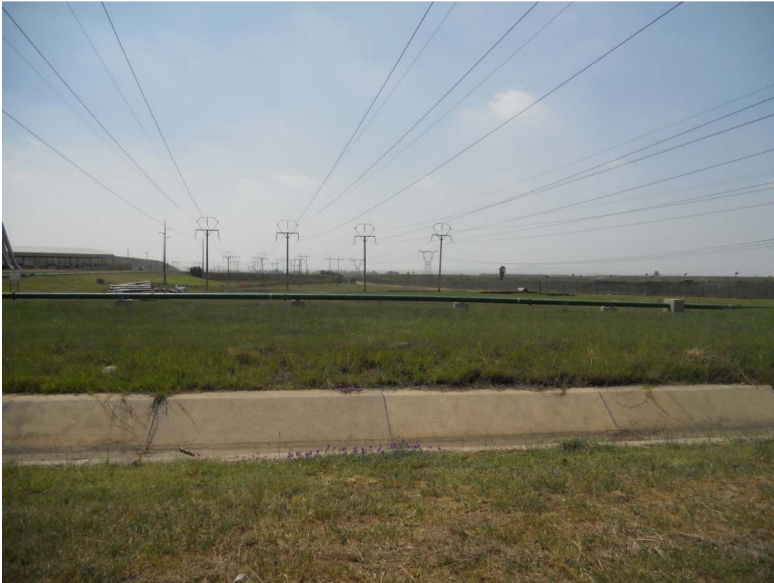
Routes C, D and F, inside the power station fence, close to the relay station, looking from west to east.
