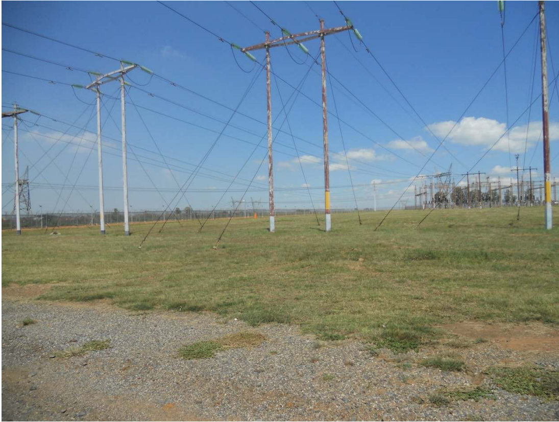
Routes C, D and F, inside the power station fence, close to the relay station, looking from east to west.
