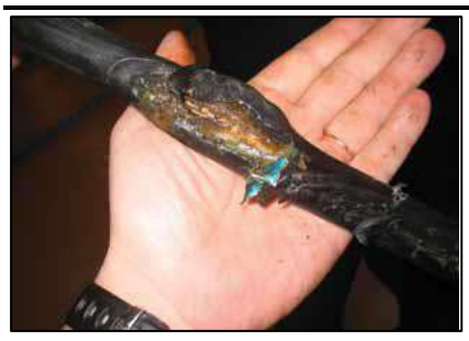
Figure 9.8 Photograph of cable damaged by a grapnel intended to retrieve fish traps from 1800 m depth.
