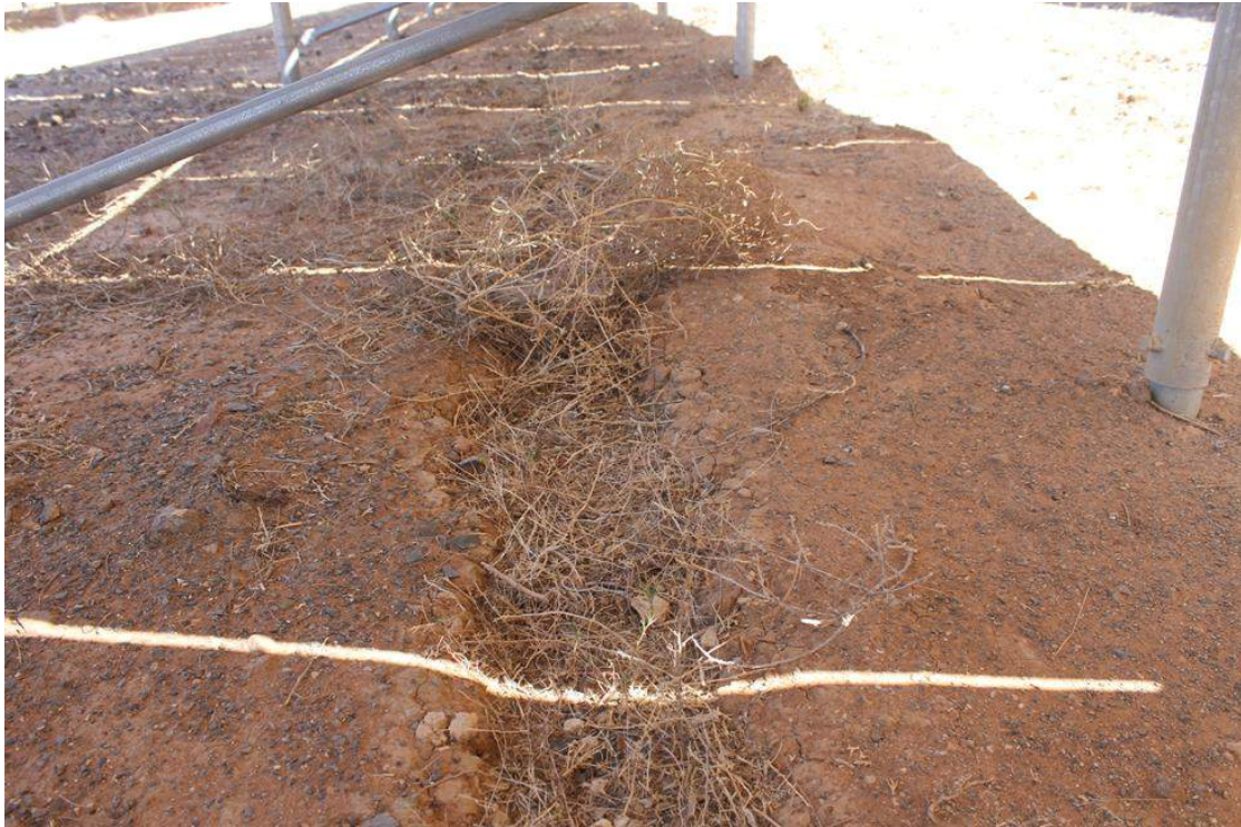
Figure 20. Image indicating rilling and plant invasion in rill under PV module. Habitat form and structure will change on site as a consequence of the establishment of PV modules
