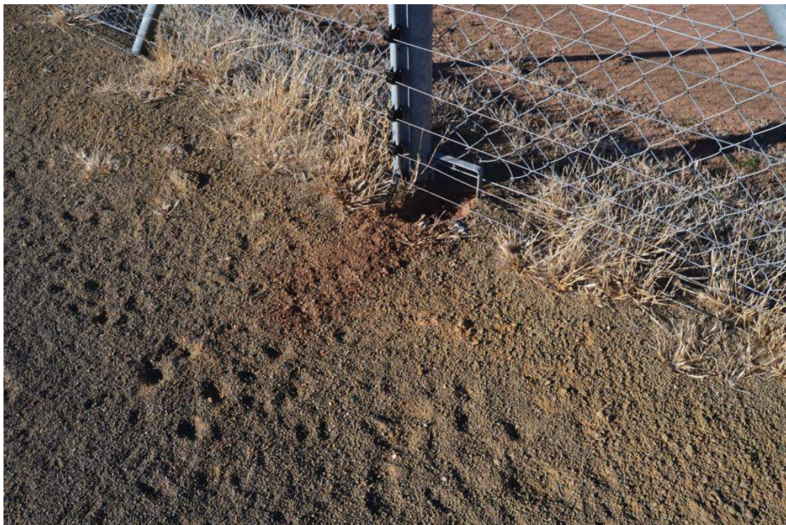
Figure 19. Image of ‘critter path’ within fence. Note spoor of smaller animals indicating use of this pathway.
