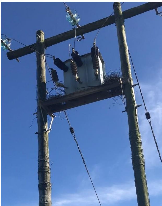
Figure 78: Crow nests constructed entirely out of wire may become a fire hazard.
