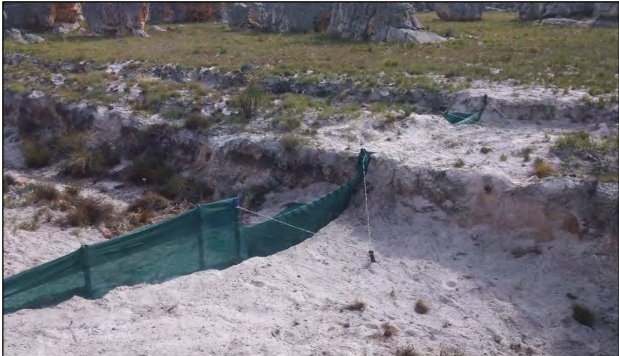
Figure 5.1: Perdevlei silt traps constructed as part of ongoing erosion rehabilitation efforts. Photo: Groot Winterhoek Field Rangers.
