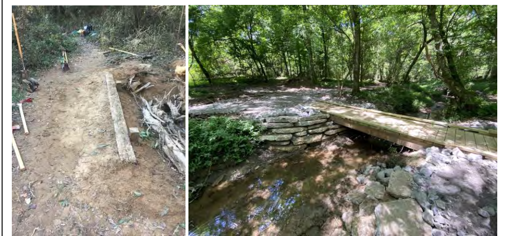
Figure 63. Retaining wall built along trail at Frenchtown Conservation Area to help stabilize trail and prevent erosion (left) and a retaining wall built with rock for stabilizing trail and stream channel along the Poplar Pine Loop trail at Forest Community Park (right; Source: BREC Staff).
