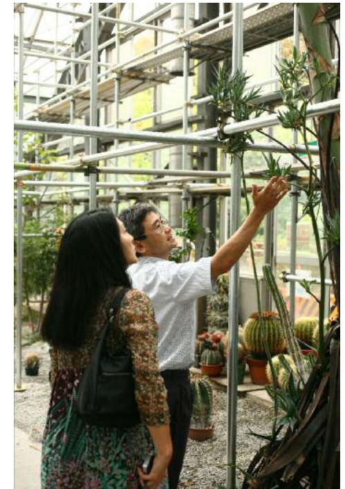
Dr Yukawa in the Tsukuba Botanic Garden greenhouse damaged by the March 2011 earthquake
