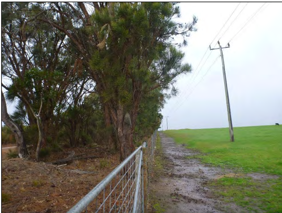
Figure 11-1: Existing 22 kV overhead power lines on Project Site (parallel to Down Road South)
