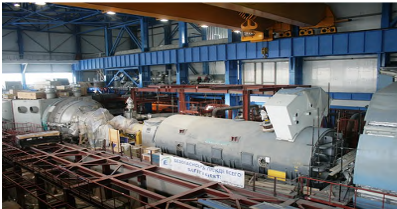
Figure 7: Sample of the Combined Cycle Gas Turbines with a capacity of 1600 MW
