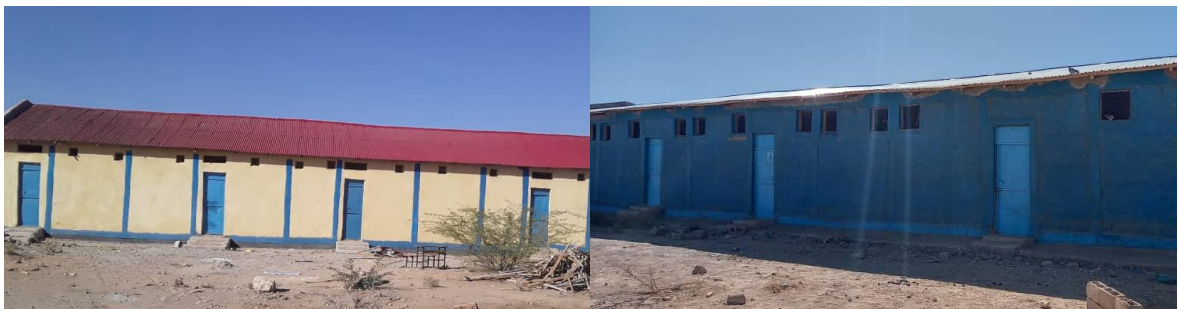
Photo 14: View of School Buildings Affected by the TL: Raho Primary (right) & Dikse Sere Secondary School (left)
