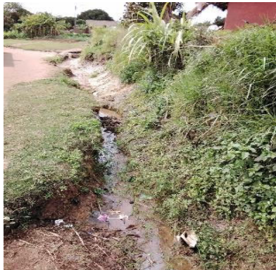
Example of erosion in Bairro 5
