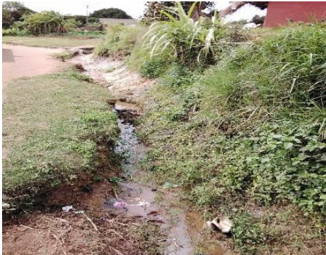
Rainwater drainage channel in Bairro 5
