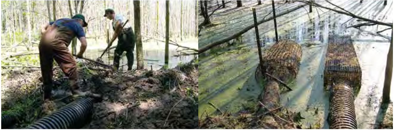
Figure 24.3 Beaver baffle control system
