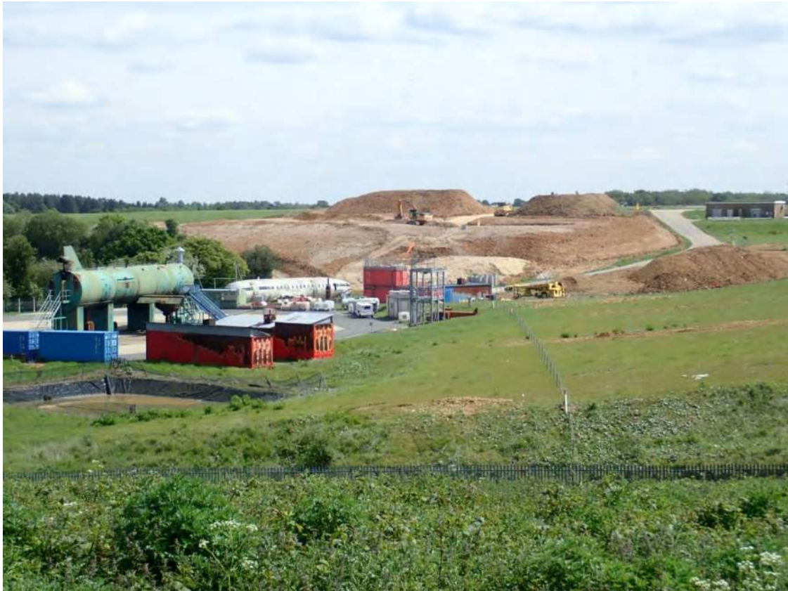
Figure 25: Fresh earthworks near the north-eastern periphery of the airside zone in May 2019.
