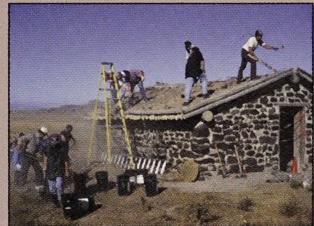
A stabilization project at Simpson Springs, Utah, along the Pony Express National Trail.
