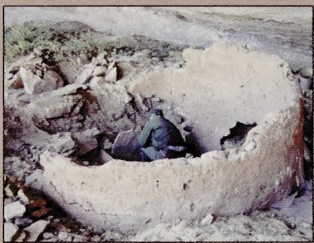
Stabilization of a masonry storage room, dated around A.D. 900, Grand-Staircase Escalante National Monument, Utah.
