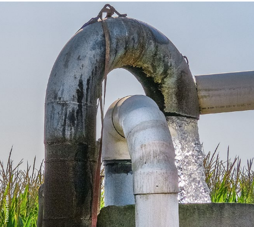
Kings County well pumping into an irrigation system.
