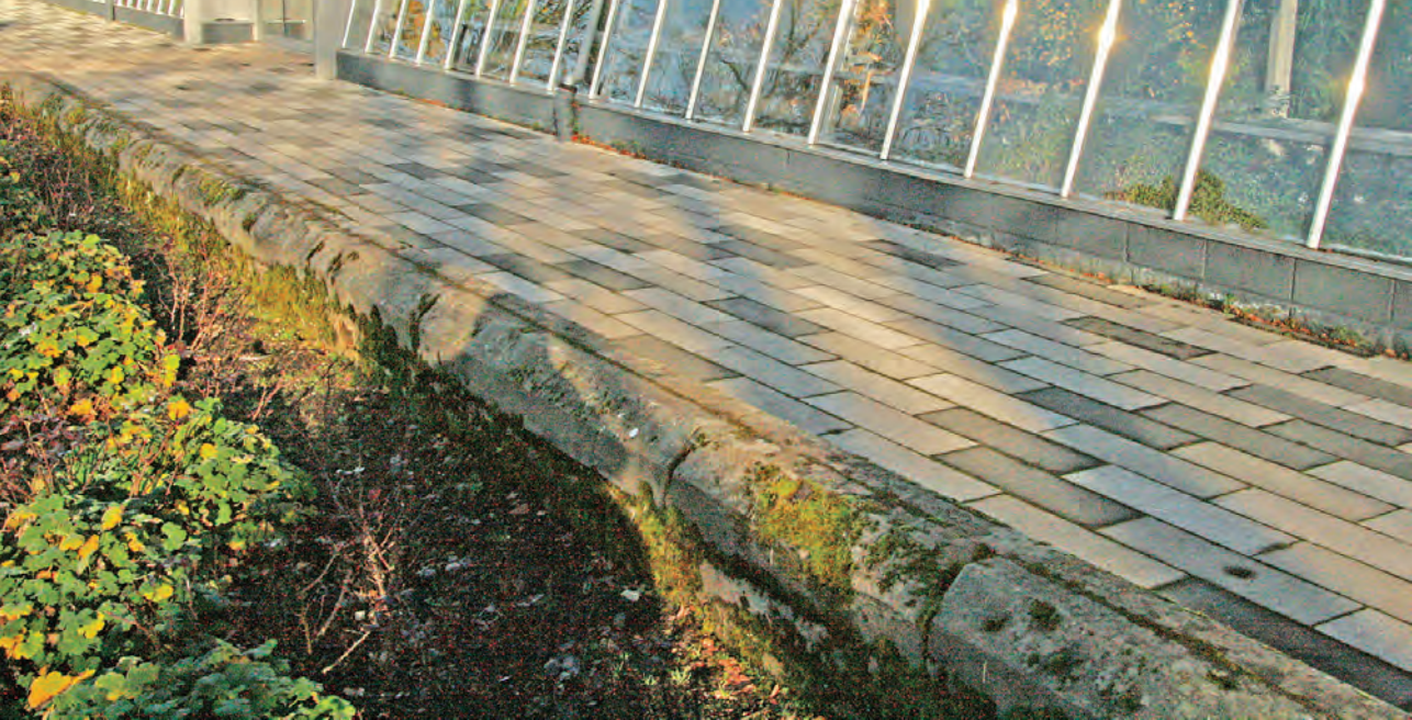
Mosses on the stonework in Saughton Park. All photos © David Adamson.
