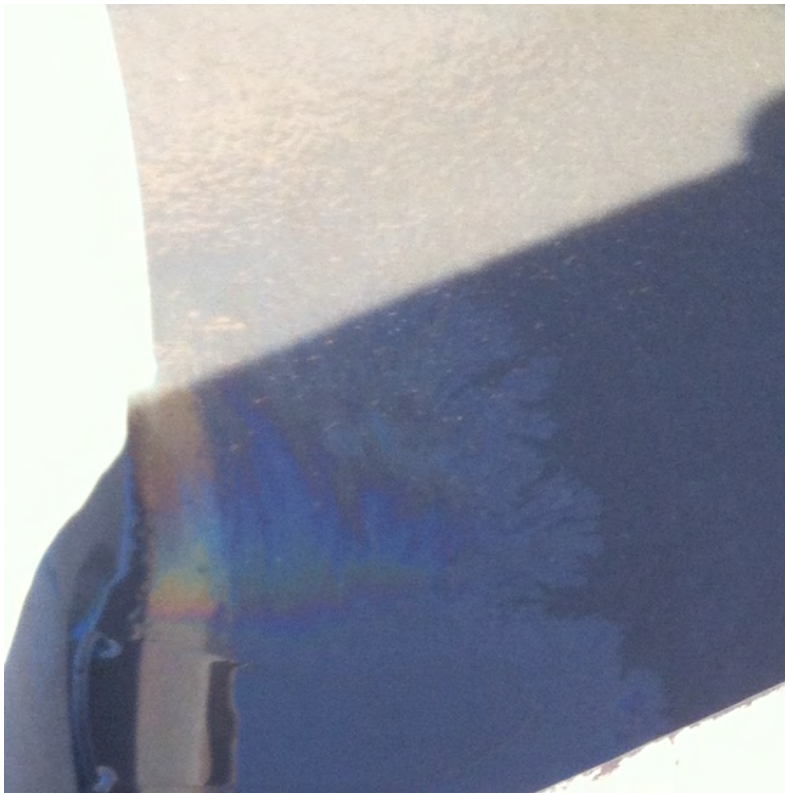
Photo 15: Oily sheen on the liquid in the secondary containment structure of the onsite waste storage tanks. Photographer: Kristen Kochelek
