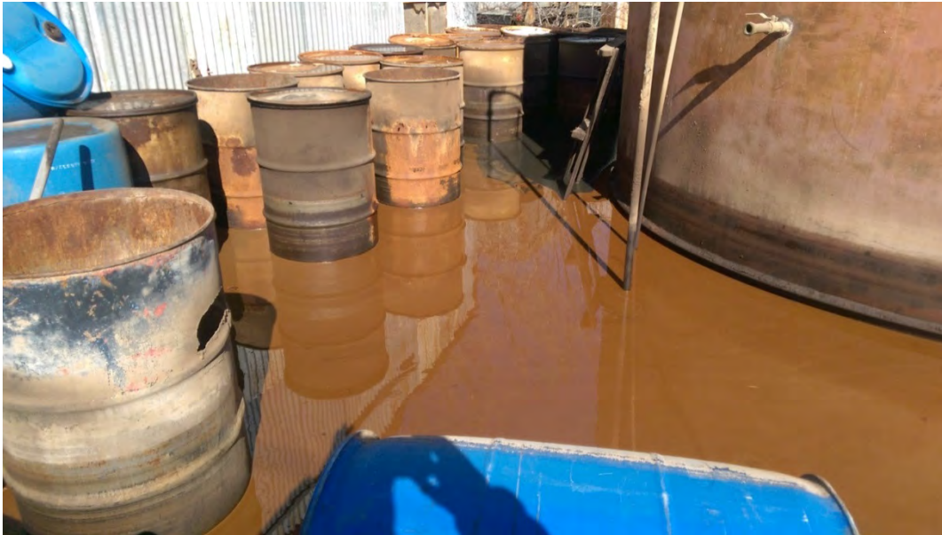
Photo 9: Plastic and metal drums in a liquid in the secondary containment structure of the onsite waste storage tanks. Liquid is orange with black substance originating from the metal drums. Facing northeast. Photographer: Stephen Ellis
