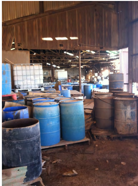
Photo 12: Inside the drum unloading area, closer to the processing area showing stacked totes, possible bulging drum, stained soil, and condition of the structures. Facing west-northwest. Photographer: Kristen Kochelek
