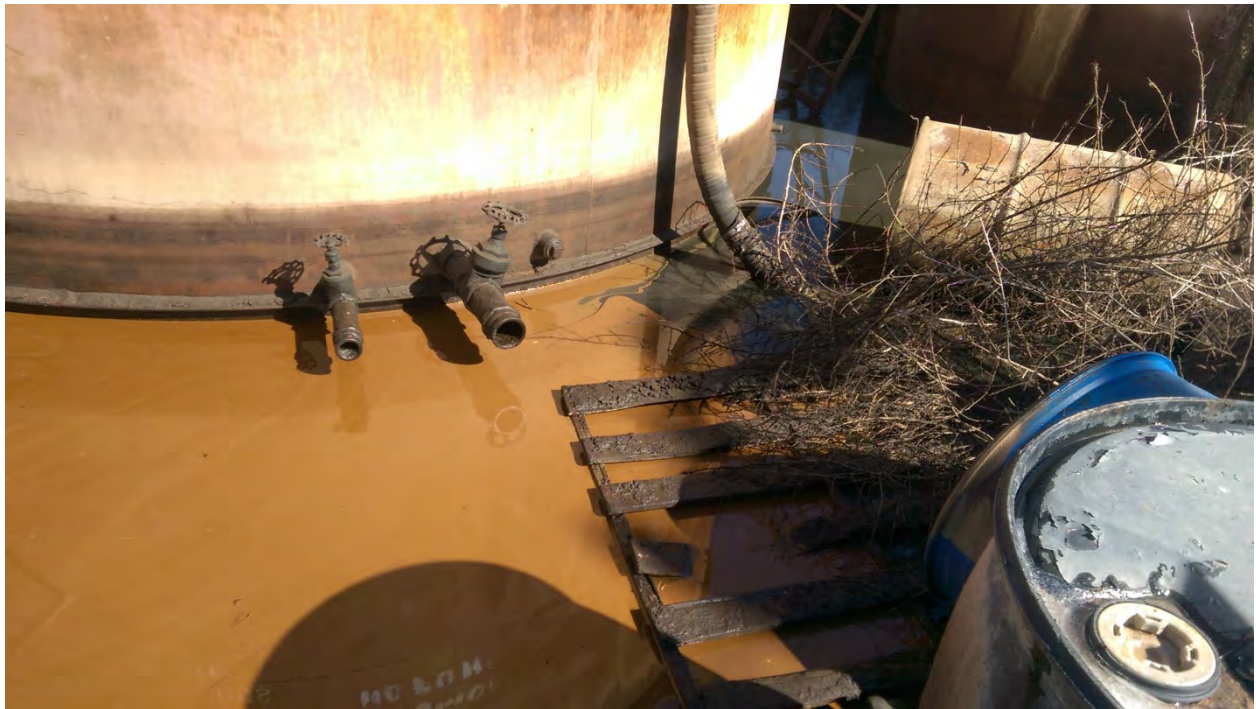
Photo 10: Debris and drums in the liquid in the secondary containment of the onsite waste storage tanks. The liquid again is orange with a black substance appearing to originate from an overturned drum. Facing southeast. Photographer: Stephen Ellis
