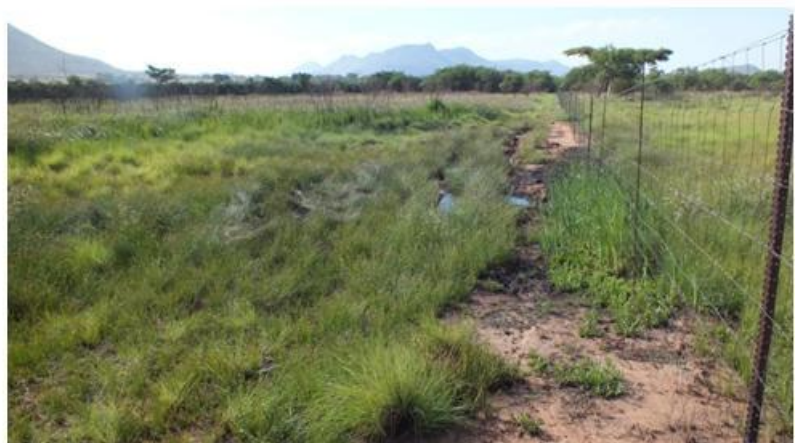
Figure 26: Some surface water prevented from draining due to the road and the canal wall.
