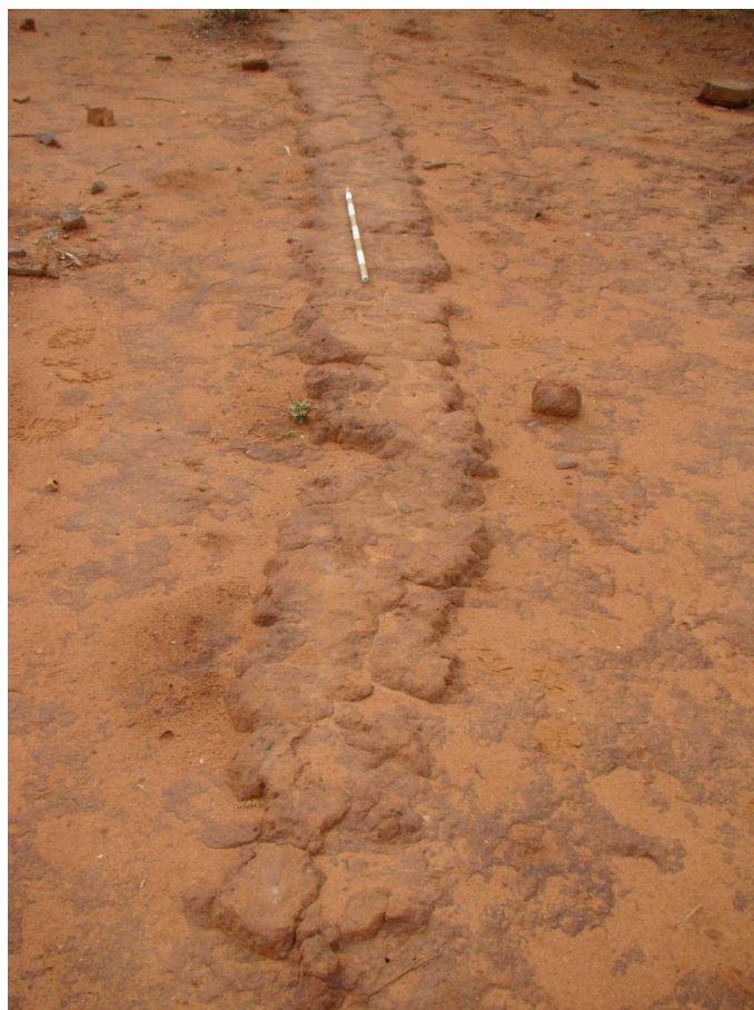
Fig. 29: Some clay foundations in the middle and southern sections are almost completely deteriorated.
