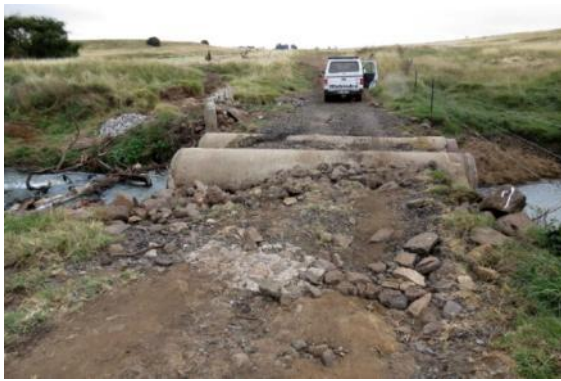
Badly constructed road through a wetland
