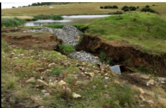
Dam with extensive erosion and dumping
