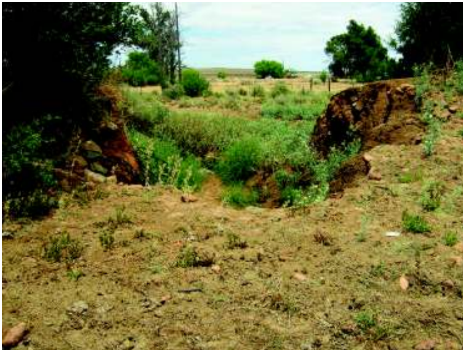
Figure 11: Badenhorst Farm Dam with a damaged embankment
