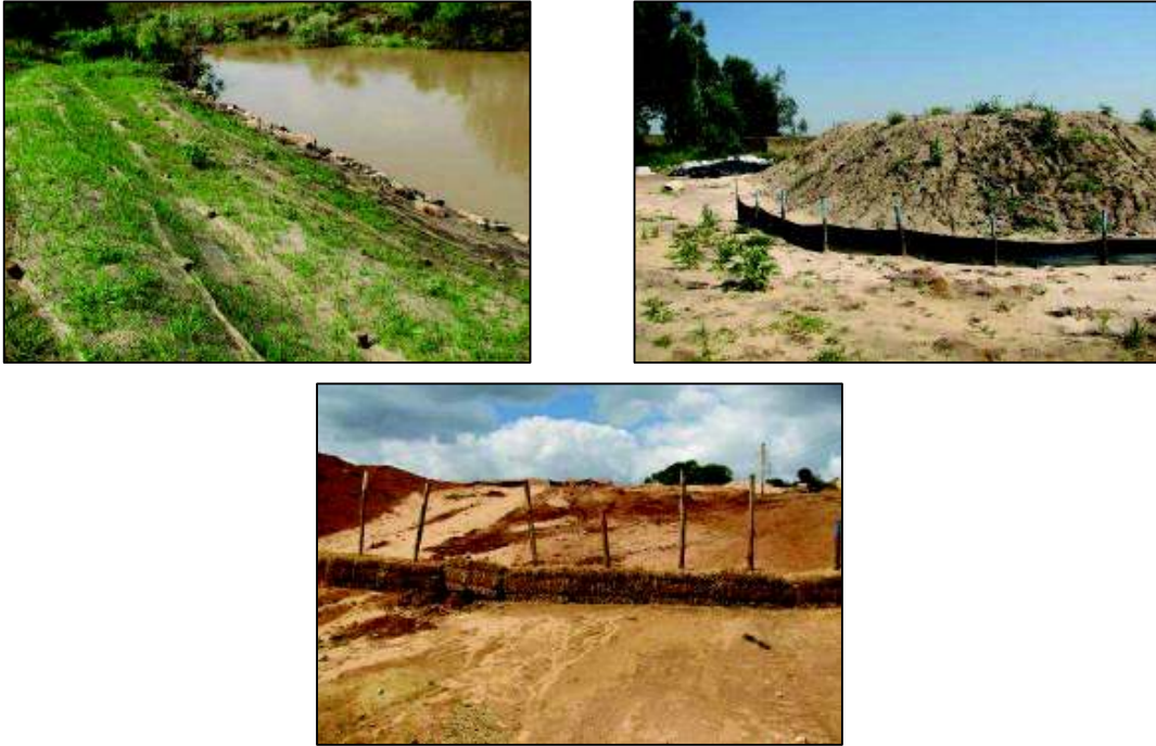
Figure 27: Typical soil erosion mitigatory measure: BioJute Installation ( top left ); a silt fence protecting a stockpile ( top right ) and pegged hay bale wall used to reduce runoff velocities ( bottom )
