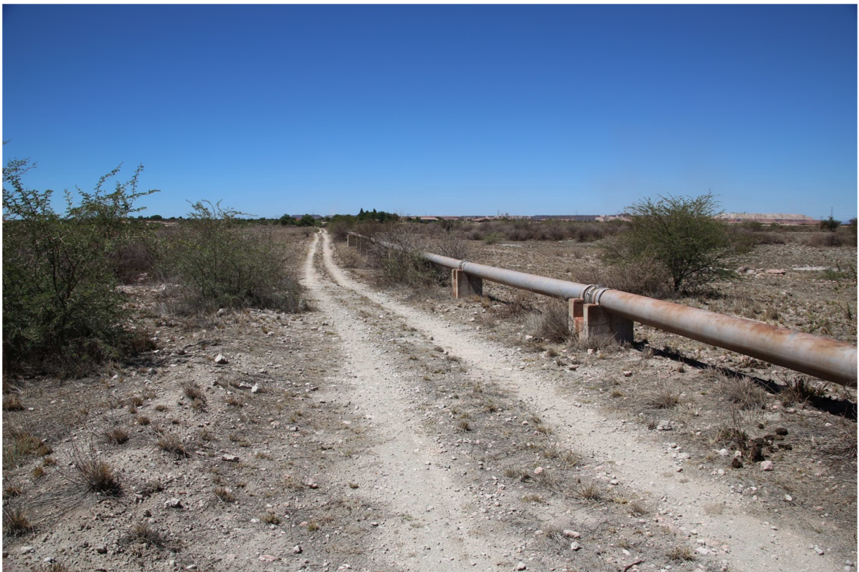
Figure A3: View of the pipeline and service road in Kathu pan.
