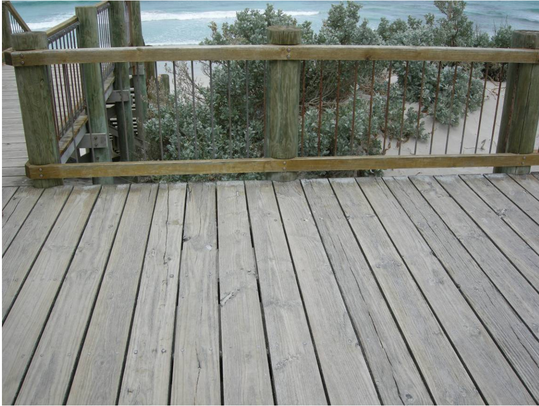
Fig. 16. View of the decking on the current Main Platform. This decking will be replaced as part of the construction.
