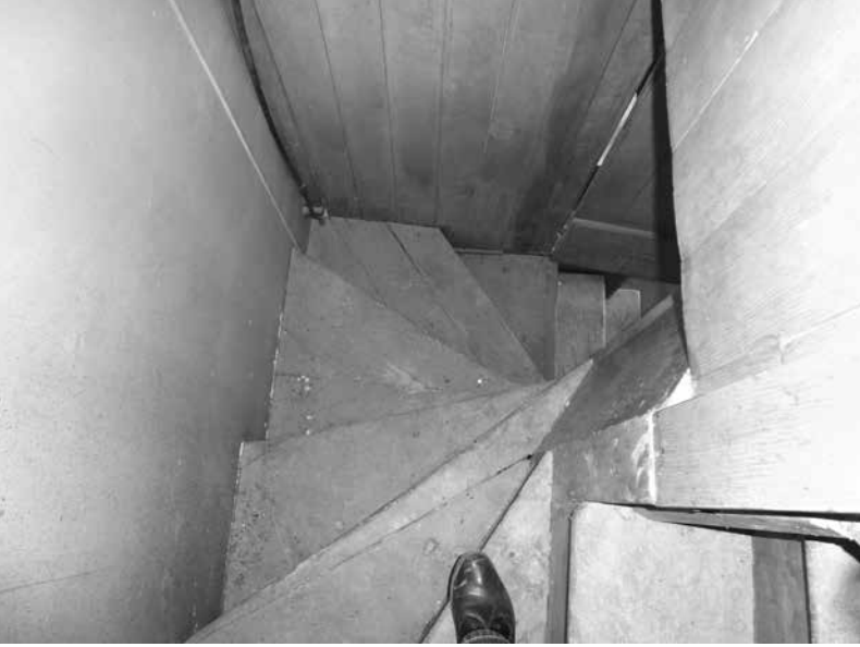
View of the U-shaped staircase of 1883 that people use to climb from the nave floor to the gallery. Every step is different, and readers can visualize from the shoe shown in the picture how narrow some of them are. Photo: Howard D. Bennett
