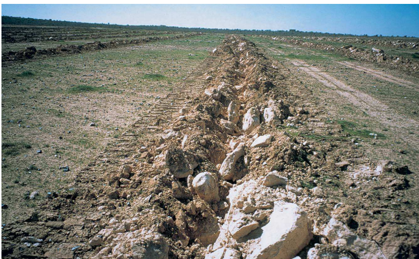
Photo no. 70. Soil preparation, ripping 60-75 cm-deep sub-soiled furrows are often mandatory in shallow soils having a thick and hard calcrete, or, alternately in deep, very compacted and little pervious clay/loam soils in order to permit water percolation and root penetration, hence a successful establishment. This type of land preparation is a standard afforestation procedure in many arid land countries. The success of this technique, however, depends on
