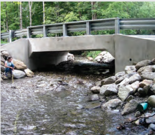
Before and After photos of an upgraded culvert using HVA best practices.
