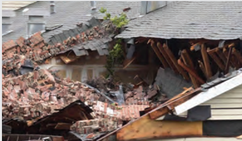
Wind damage in Bethel Photo Ctpost.com
