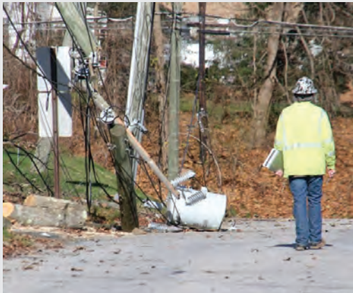
Destroyed transformer, Nov 2020 Photo: John McKenna
