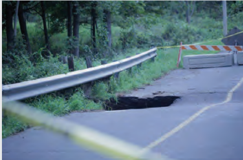
Bridge washout in Middlebury Photo Patch
