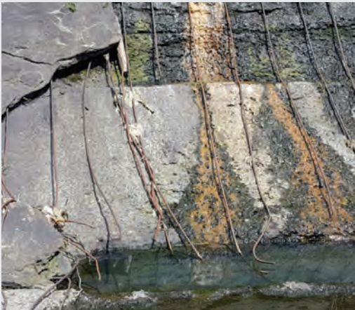
Cracks and exposed rebar on the dam J. Waldman
