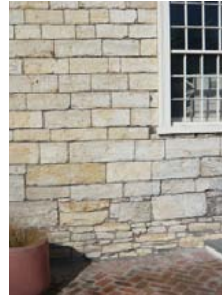
Repoint mortar joints where there is evidence of deterioration.
