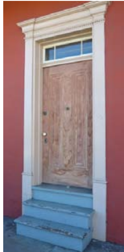
When replacing a door, use a design that has an appearance similar to the original door, or a door associated with the building style or type.
