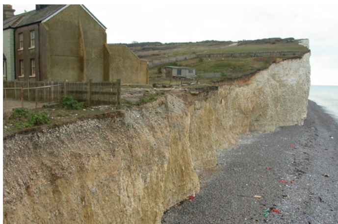
Coastal erosion and "head" deposits at Birling Gap: Photo Ken Merrifield
