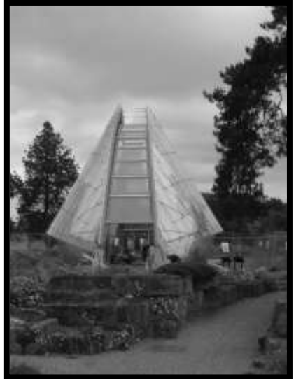
The new alpine house at Kew Gardens under construction in May 2005. Photograph by Paddy Tobin
