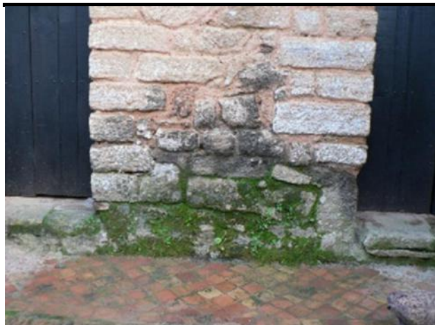
Fig.9: Colonization of the base of a calcarenite wall in Chellah by bryophytes thanks to the capillary rise that favors a high degree of moisture
