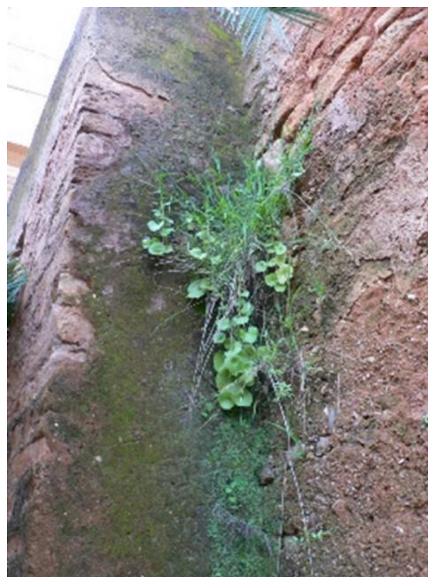
Fig.8: Terracotta brick wall of the gate covered with bryophytes that maintain a high degree of moisture on the masonry
