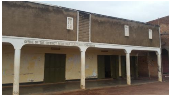
current office of the District Registrar Source: Last Mile ESIA Field Photos 2017
