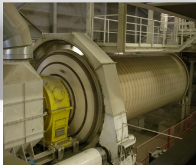
Conditions during the cement grinding process
