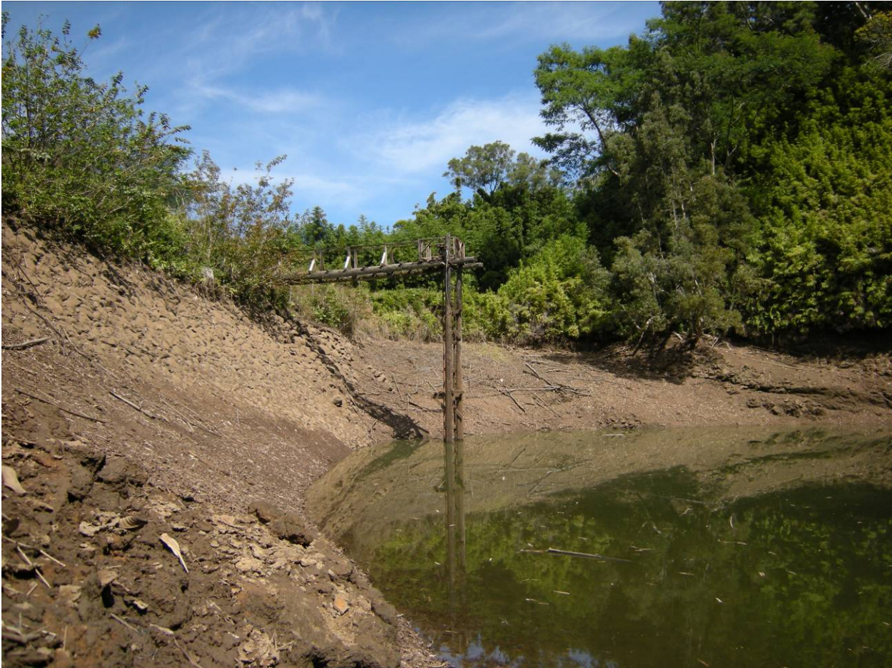
Photograph 2. HI_ Maui County_Kolea Reservoir_2. Catwalk and upstream slope of the dam showing the rip rap section. View facing north.
