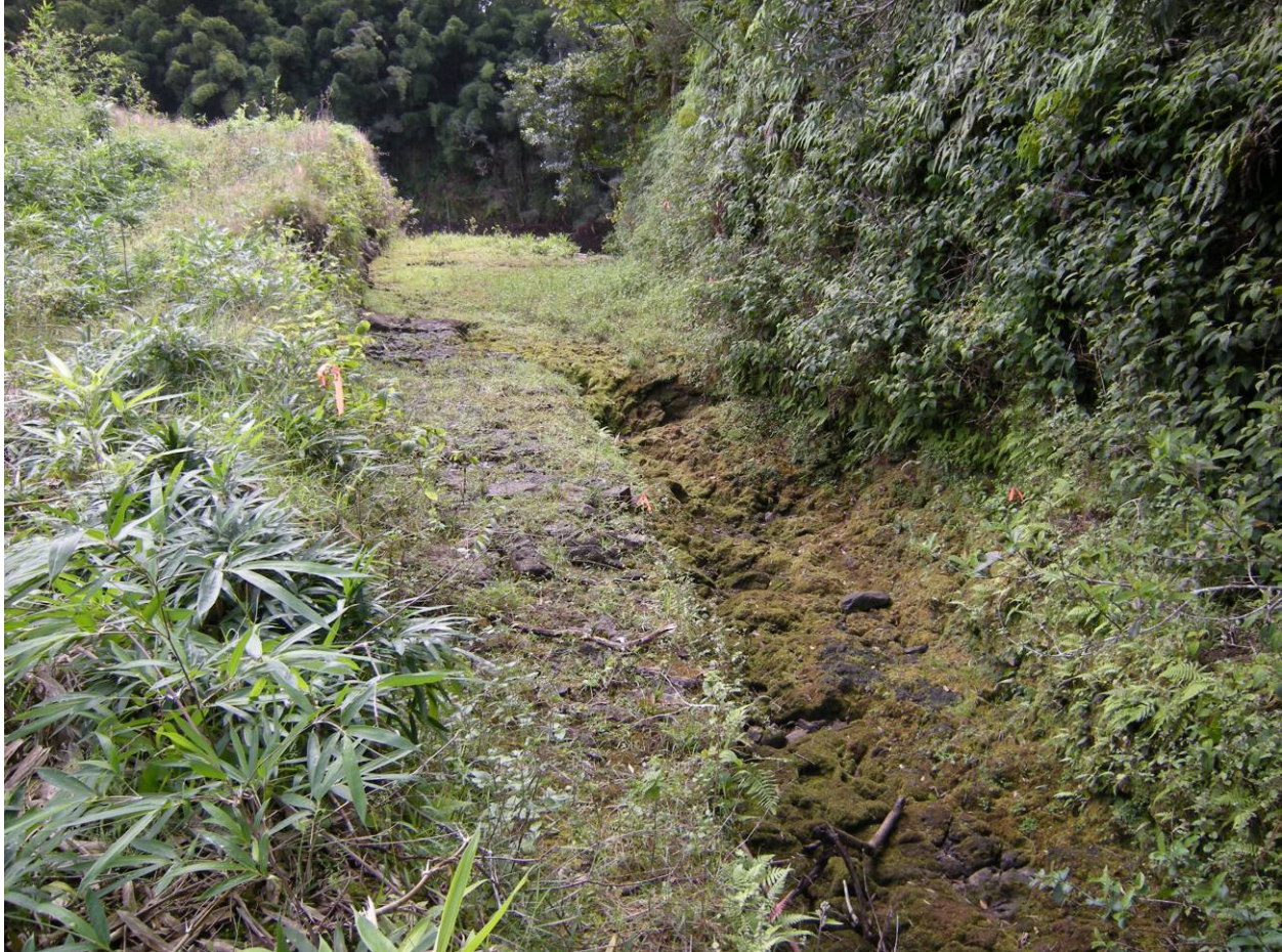
Photograph 5. HI_ Maui County_ Kolea Reservoir_5. Spillway cut into the rock at the south abutment of the dam, with the spillway inlet in the background. Note the narrow natural gully at the lower right. The basin of the reservoir is in the background, the dam extends to the left View facing southeast.
