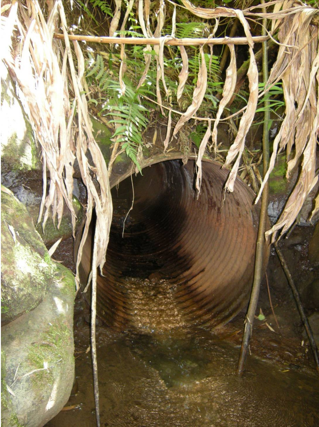
Photograph 7. HI_ Maui County_Kolea Reservoir_7. Detail view of the visible portion of the outlet works at the downstream toe of the dam. View facing southeast.
