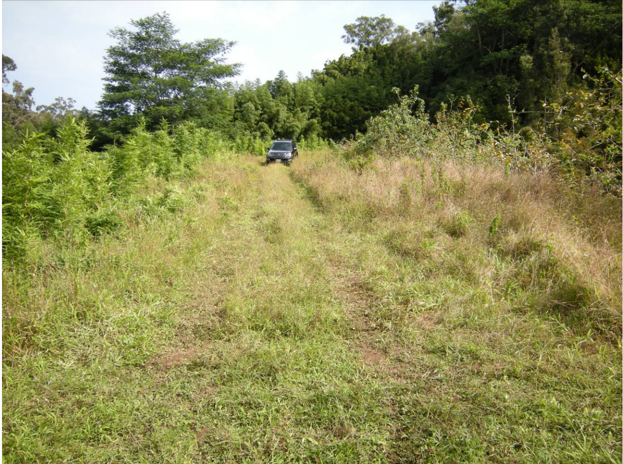
Photograph 4. HI_Maui County_Kolea Reservoir_4. The crest of the Kolea Dam. The vehicle is parked adjacent to the catwalk. View facing northeast.
