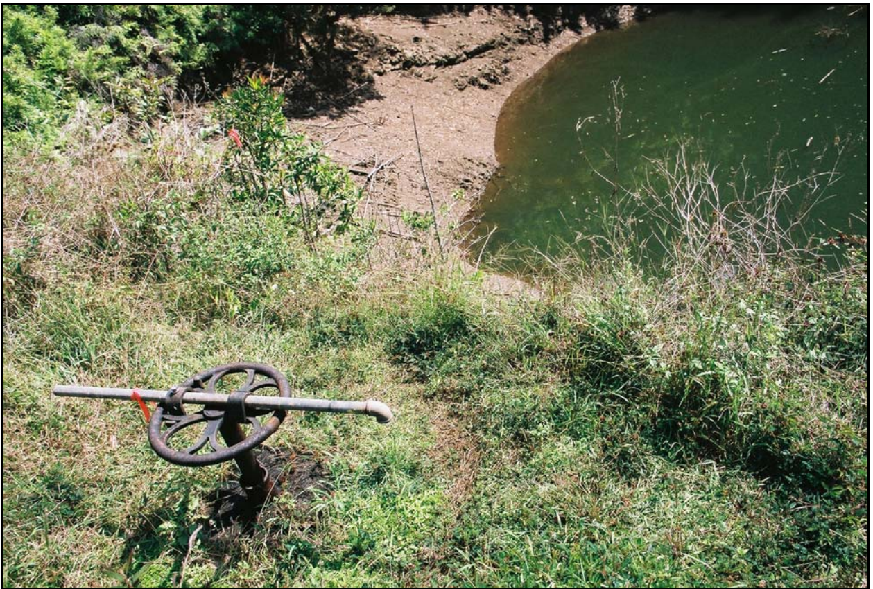
Figure 17. The secondary outlet valve control for Feature E, view to the north.
