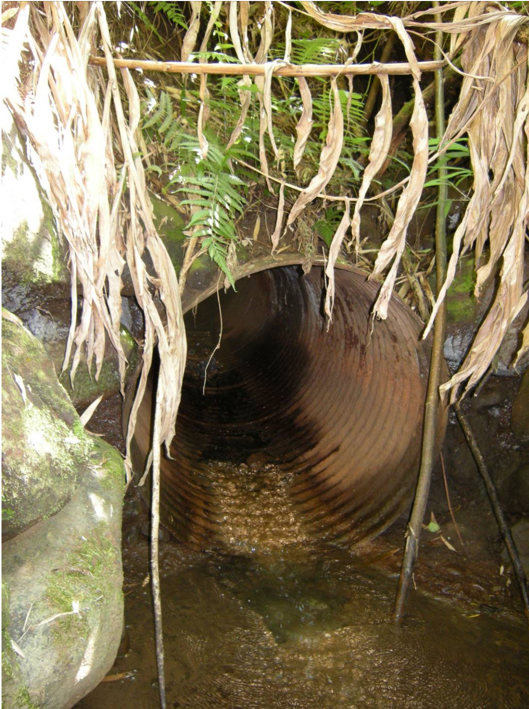
Photograph 7. HI_ Maui County_Kolea Reservoir_7. Detail view of the visible portion of the outlet works at the downstream toe of the dam. View facing southeast.
