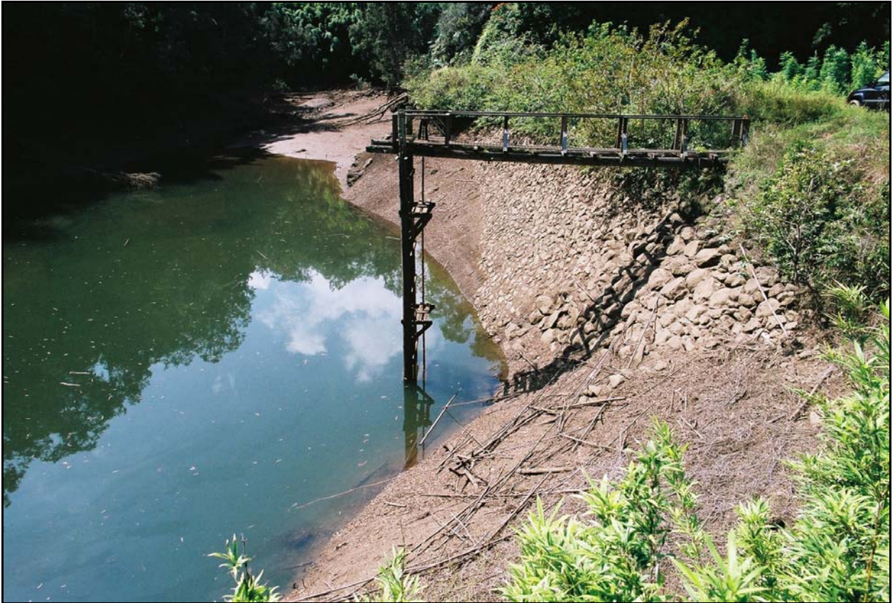
Figure 15 Feature B, the catwalk, and Feature C, the reservoir, view to south.
