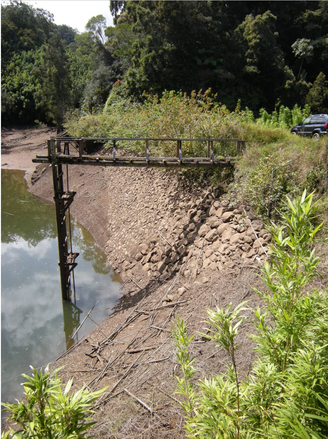
Photograph 3. HI_Maui County_Kolea Reservoir_3. Catwalk and upstream dam embankment showing the rep rap section. Note the outlet valve shaft extending down just to the right of the vertical pole supports of the catwalk. View facing south.
