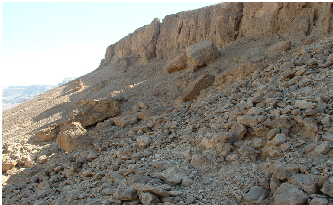
Plate 5.14. Association 5.5.10. Very eroded and unstable steep slopes with vegetation cover less than 2%. The vegetation is mainly found in runnels and rills.
