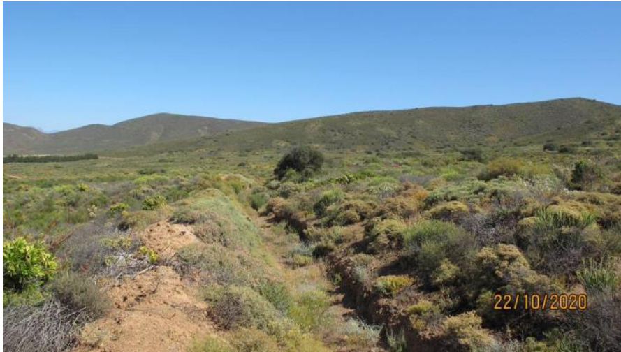
Photo 5: The cut-off trench in the northern portion of Area 1 (looking from east to west along the trench).
