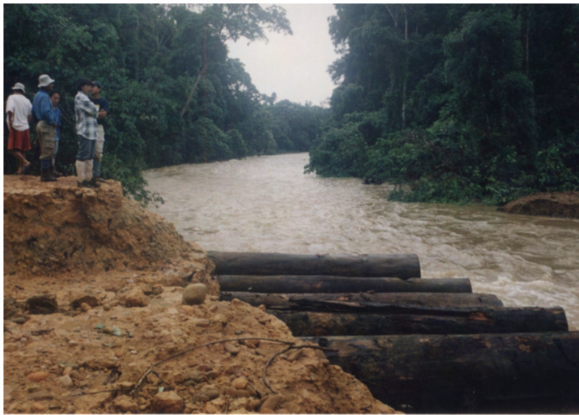
Figure 7. Accessibility to the primary forest plots. The above photos showed a broken bridge due to sudden flooding a night before.
