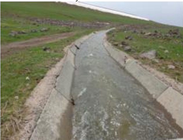
Water Transfer to Reservoir through Geghardalich Derivation Canal
