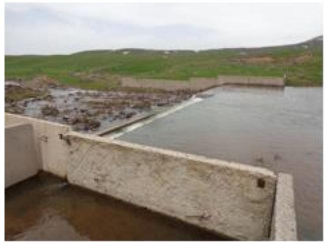
Intake Structure for the Derivation Canal
