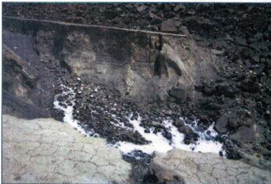
Photo 14. Seepage springs on the downstream side of the dam causing erosion of the debris-flow (i.e. flood-plain) deposits lying on the blocky dam material to the right (bottom of photo). Photo credit: Jörg Hanisch.
